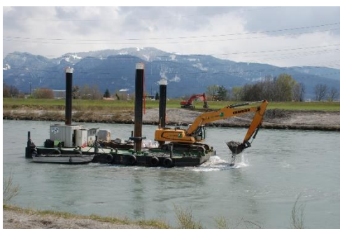
Figure 1: Artificial de-clogging of the Alpine Rhine river by excavating the river sediments.
